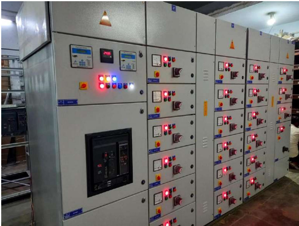
AUTOMATIC POWER FACTOR CORRECTION (APFCR) PANEL
