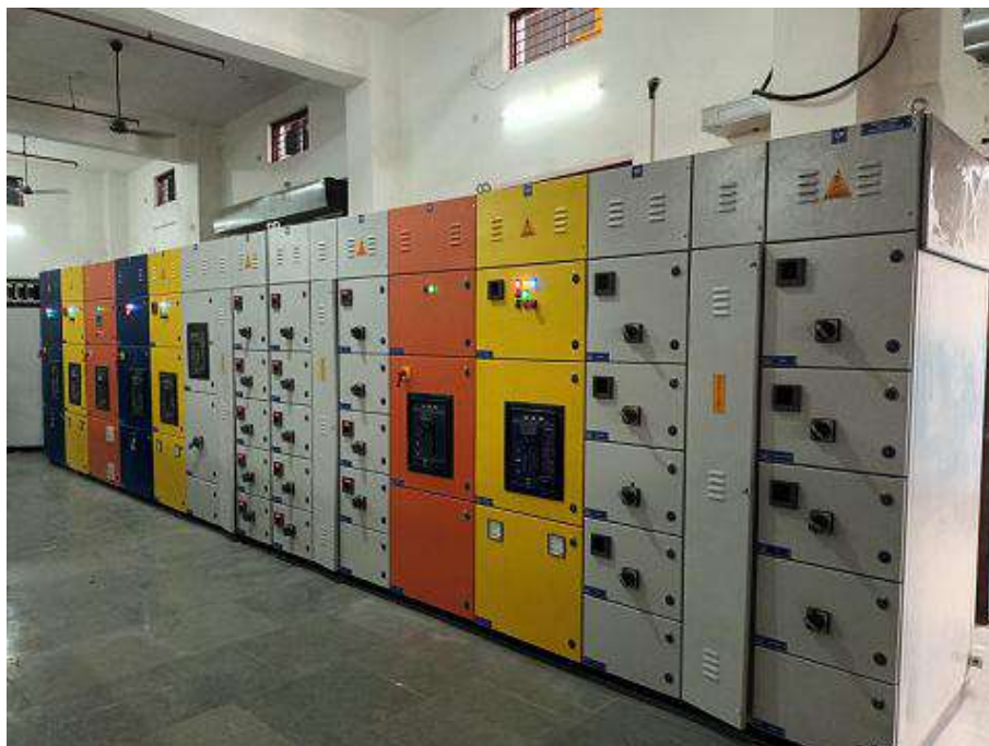
POWER CONTROL CENTRE (PCC) PANEL
