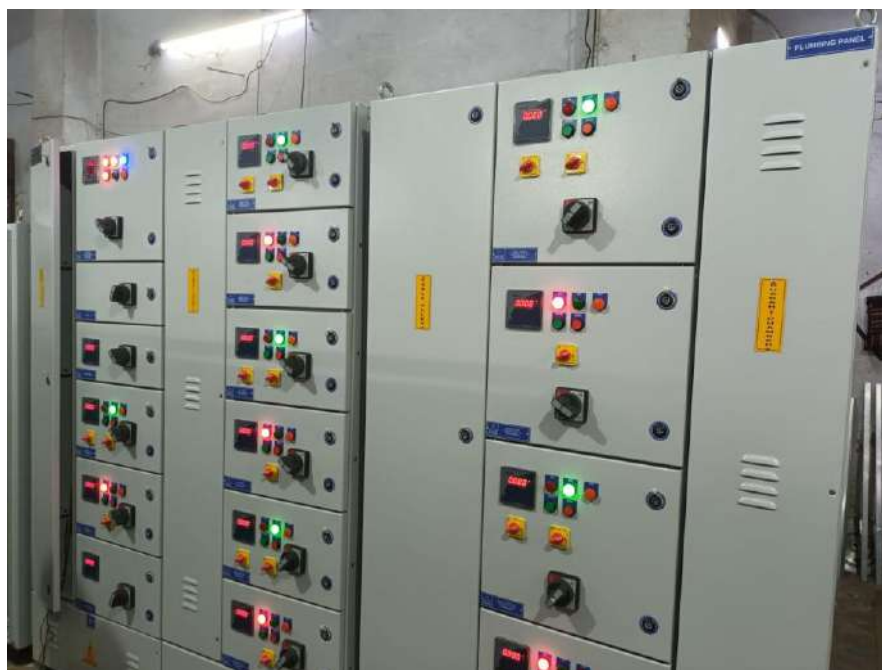
MOTOR CONTROL CENTRE (MCC) PANEL
