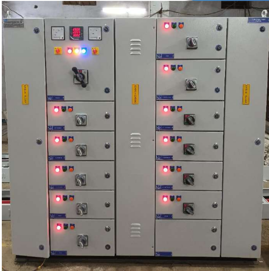
POWER DISTRIBUTION PANEL / PDB PANEL
